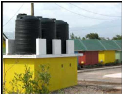
Water Storage tanks for Fishing Village
